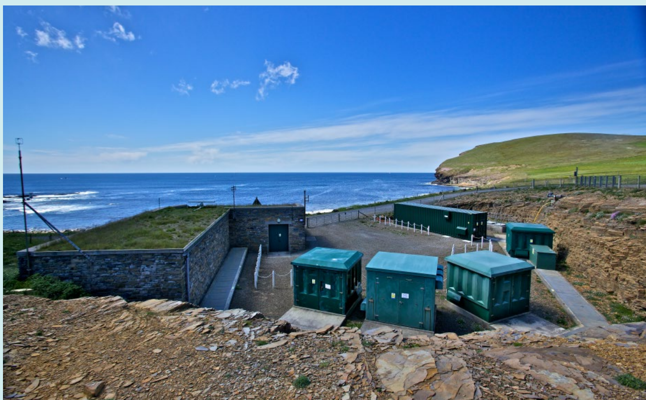
EMEC Billia Croo substation (Source: EMEC, Colin Keldie)
